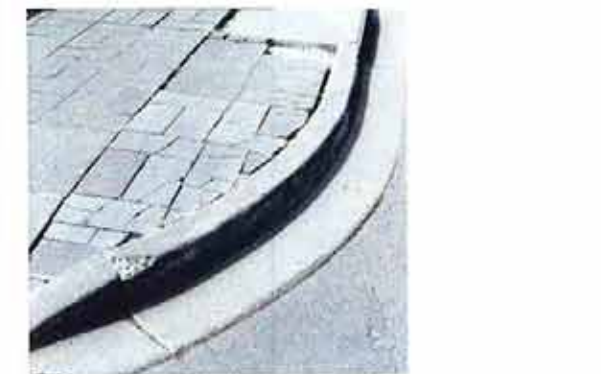
Existing Surface in poor condition
